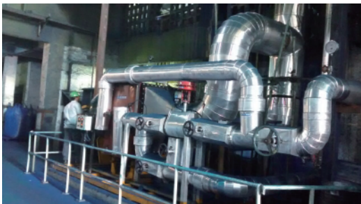
Industrial Heating Equipment
